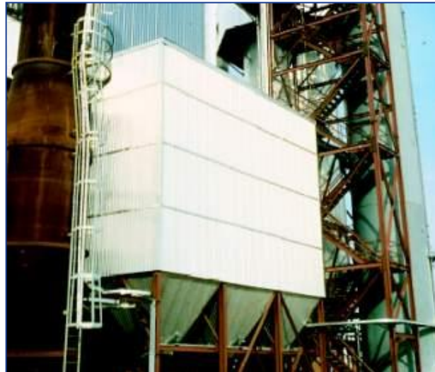
Coal-fired Industrial Boiler 110,000 ACFM
