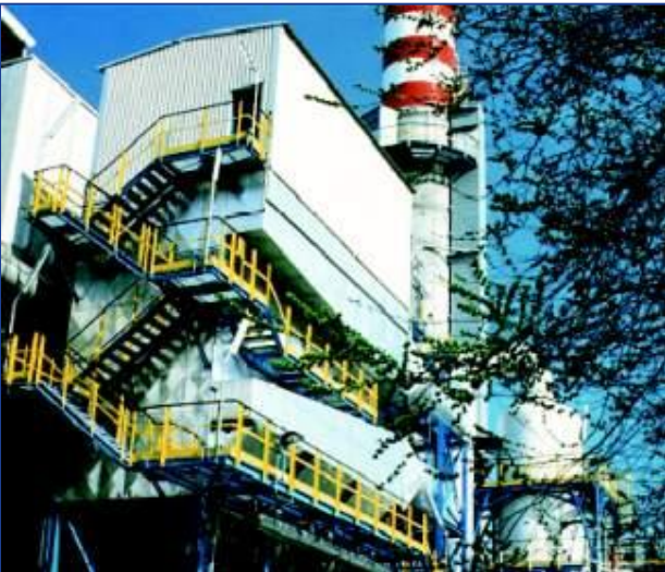
Municipal Solid Waste Incineration 16 MW – 65,000 ACFM
